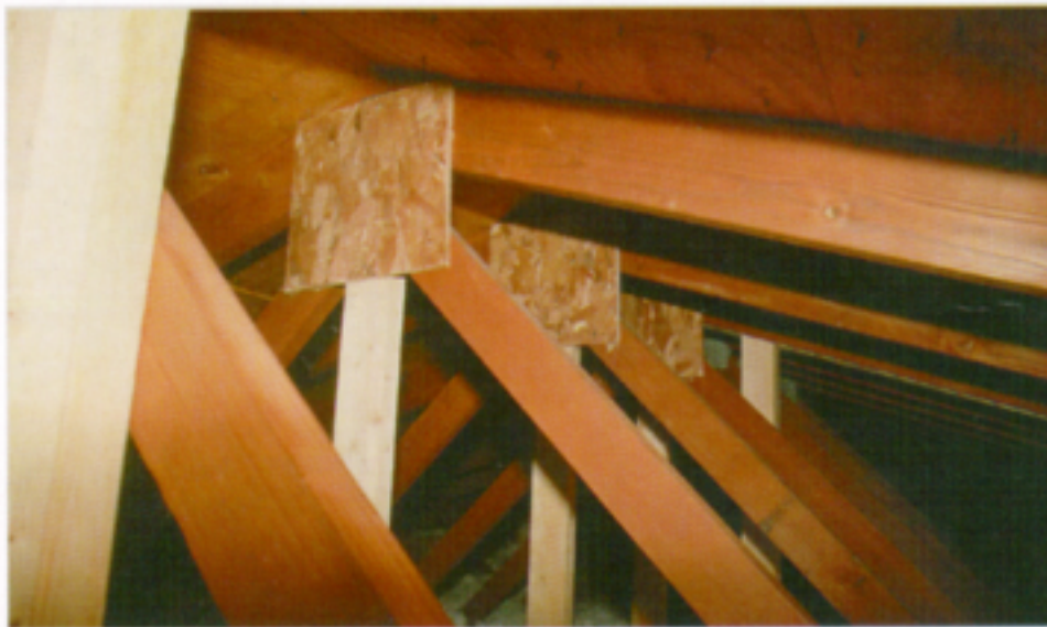
Figure 1. The first step in modifying the truss roof structure (top) was to add support posts from the peak to a bearing wall below (bottom). OSB gusset plates secured the connection.
