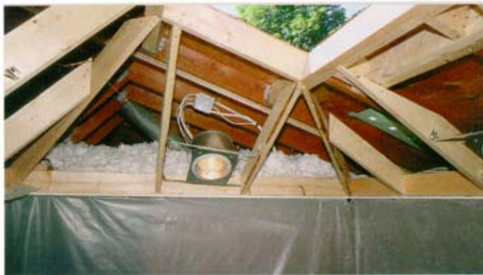
Figure 4. Recessed lights in the skylight well make it an important source of light and a visual focal point at night as well as during the day.
