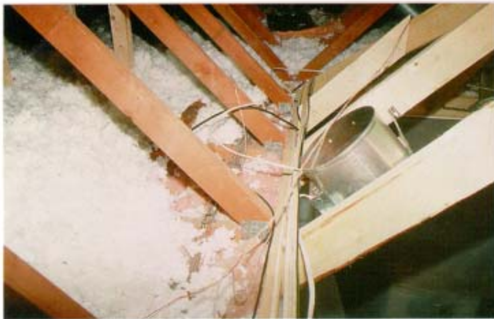
Figure 3. Cutting the bottom chord of the truss a little beyond the metal plate allowed the original truss web to provide some support for the drywall ceiling.
